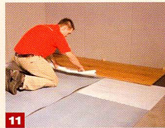
11 The second parquet section is pushed into the first until it locks in tightly (seamless); following this, the auxiliary film between Elastilon and the parquet board(s) is removed. From now on, work is carried out with the actual protective layer of Elastilon.
