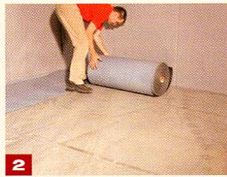
2 Roll out the Elastilon over the polyethylene film in strips that lie next to one another (the strips must not overlap)
