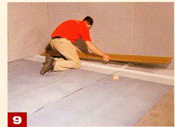
9 The first parquet section or board is now positioned on the auxiliary film.
