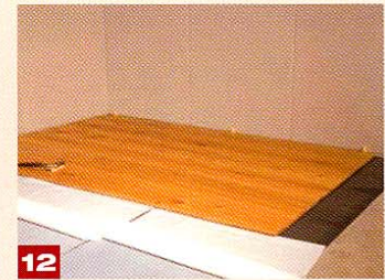
12 From here onwards, several boards can be positioned seamlessly before the protective layer between the wood and the Elastilon is removed.
